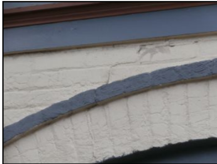
Normal settlement cracking in brick present
