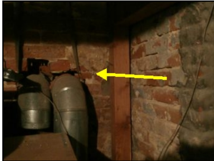
Settlement Cracking present
