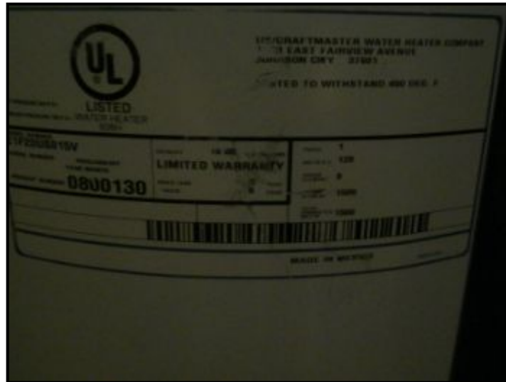
Water heater in attic
