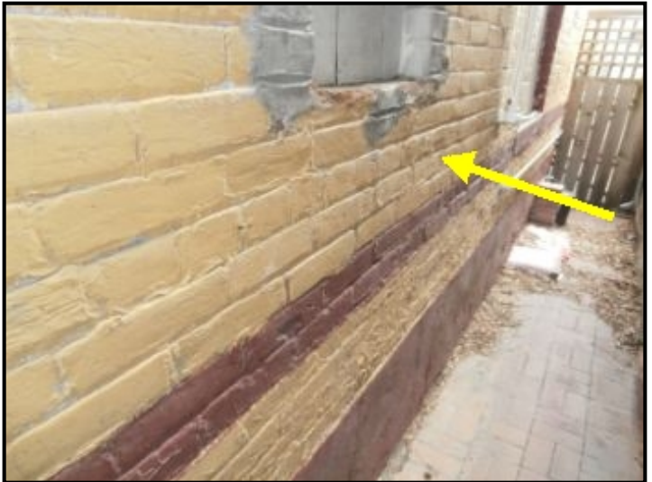
Paint on west and east sides is peeling
