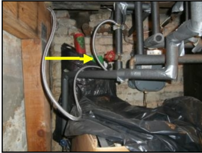
Water main shut off - basement on north wall
