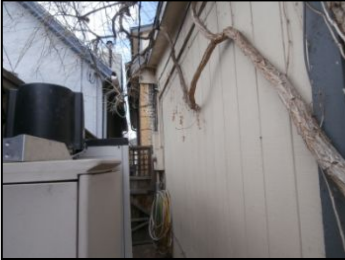
Plants are close to electrical wiring - should monitor
