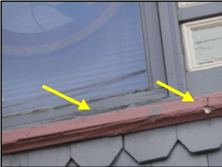
Some paint and caulking in need of repair
